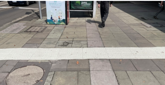
5 Footpaths are uneven and inconsistent, and some paving gets slippery when wet.
