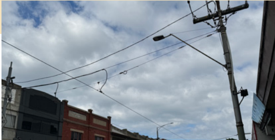
4 Existing lighting caters for the road with a lack of pedestrian level lighting.
