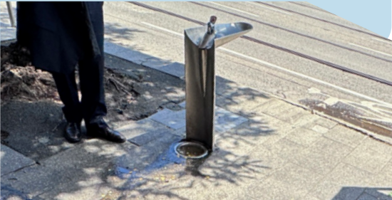
4 Minimal access to public drinking water (only one public fountain identified).
