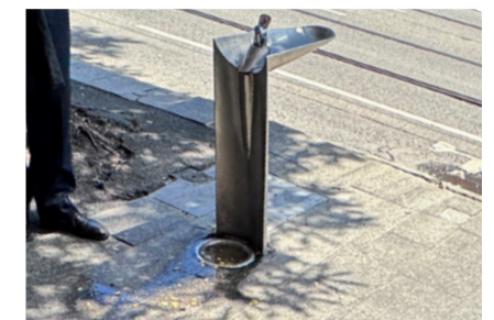
Existing drinking fountain
