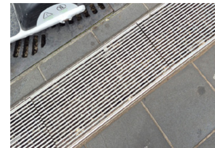
Existing drainage grate
